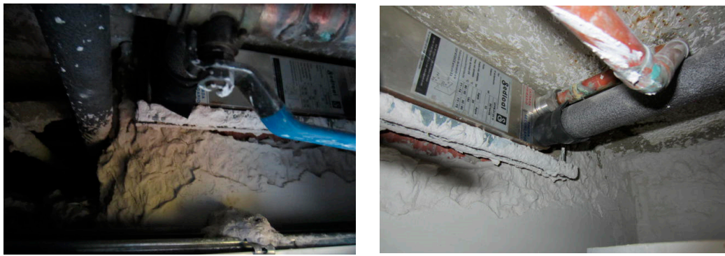
(b) An individual heat exchanger for a solar domestic hot water (DHW) system (secondary communal circuit)
