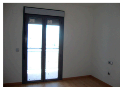
(f) The airflow across service penetrations: electrical outlets
