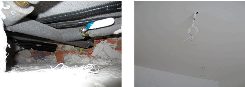
(c) The discontinuity in a lowered ceiling generated by a penetration for an electrical conduit
