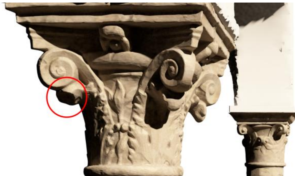
Figure 10. Defect in column capital 5 (ID tag in HBIM: Capital_5 ).
