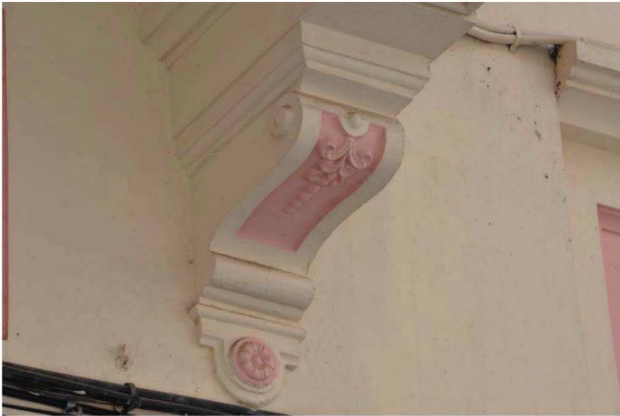
Fig. 9 Balcony bracket of the building nº 57 of Castillo Street. S/C Tenerife
