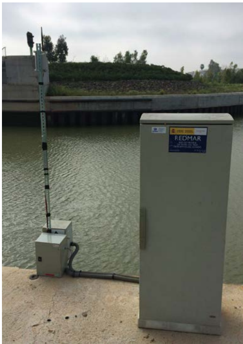
Figure 4. A sensor for tide height installed in the “Gate of the Sea” lock at the entrance of the Port facilities in the city of Seville. This sensor is wirelessly linked to the integration platform.
