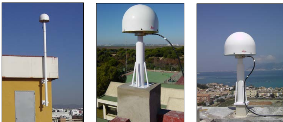
Figure 2: CRDB station, UCAD station, ALGC station.
