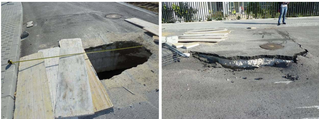
Figure 10. Damage arising from soil subsidence in the exterior area around the building and on the perimeter access roads.
