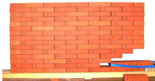
Figure 8. The wall after collapse.
