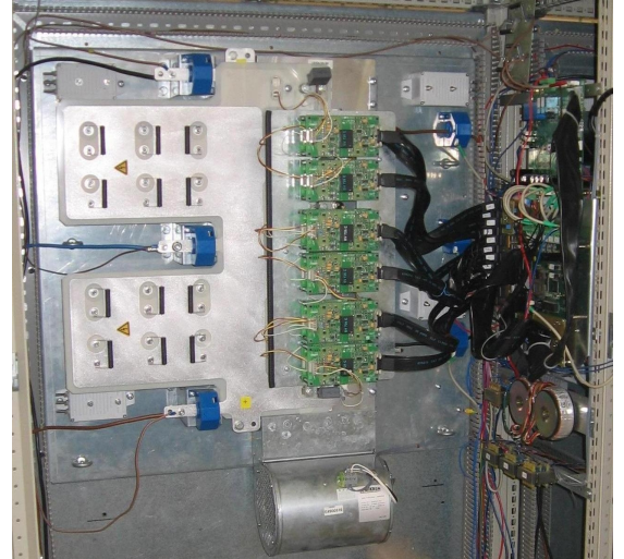
Fig. 2. 150 kVA IGBT-based three-level diode-clamped inverter prototype.
