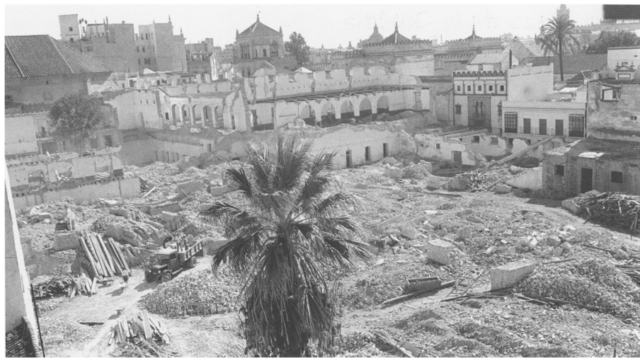
Fig. 4 Demolition of the former Jesuit School of San Hermenegildo in the location later occupied by Seville's police headquarters (Source: Archivo Serrano/ICAS)
