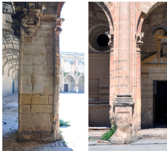
Fig. 1. Severe damages on columns of the Monastery of San Jeronimo (Seville - Spain) affected by moisture [6].
