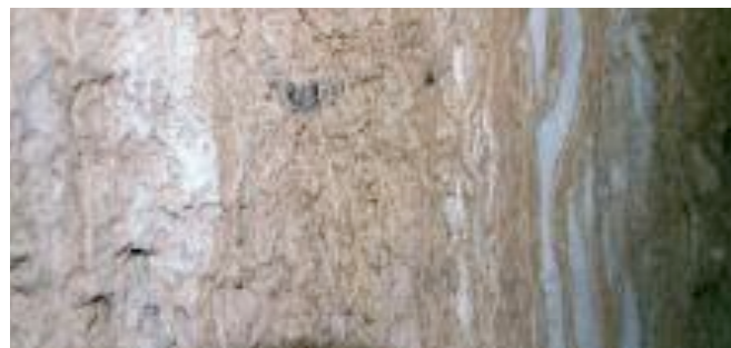
Fig. 5. Worm cast type structures visible at Ambel beneath a previously damaged roof section
