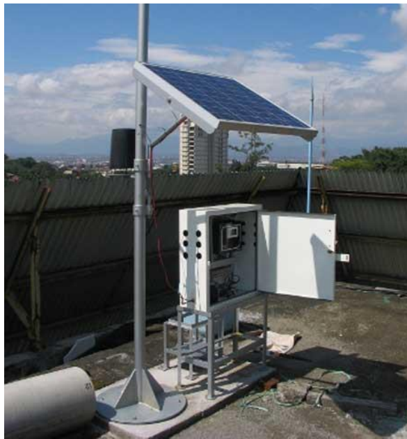
Illustration 1. Weather Station, using a data logger
