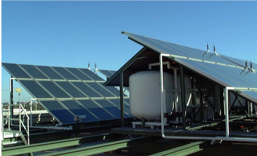
Figure 1: The solar air conditioning plant
