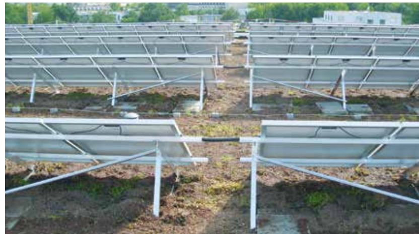
Tittmann Solar | State Theatre Stuttgart - Germany System: 112 kW | Triangle System
