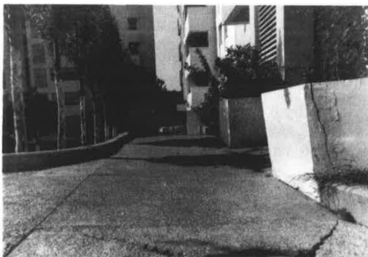
Fig. 8. Distorsions in pavement
