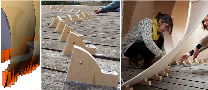
Figure 11: Left: Auxiliary sectioning planes (in vertical position) to determine the shapes of the wedges. Middle: Photograph of the definite position of the wedges after setting out with the total station and the full-scale templates. Right: installation of nylon cable ties to link the wooden surfaces to the wedges.
