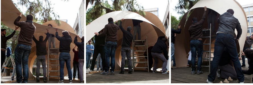
Figure 13: Left: Transportation of the unfolded surface to the installation place. Middle: Bending of the surfaces. Right: Final bending of the surface and installation of ties.
