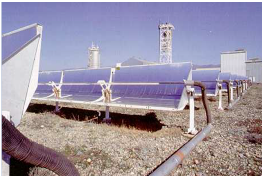
Figure 5.1: ACUREX distributed solar collector field
