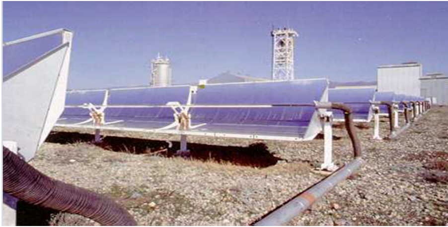
Figure 8.1: ACUREX distributed solar collector field
