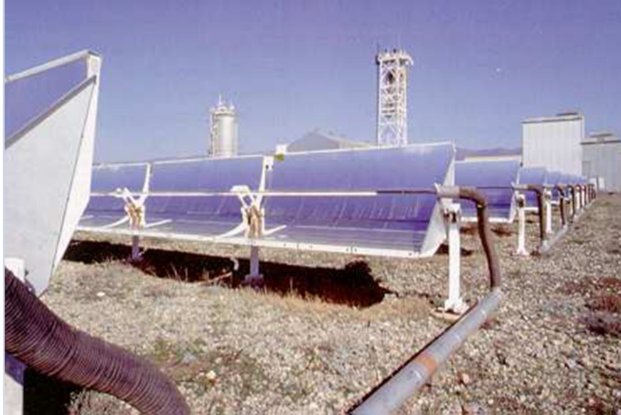
Figure 6.1: ACUREX distributed solar collector field
