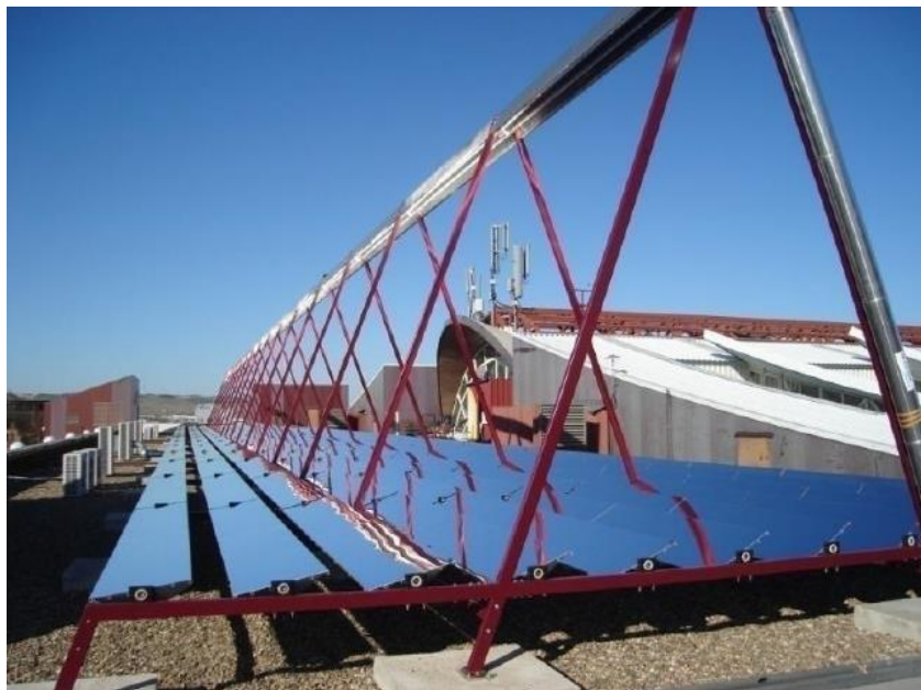
Illustration 6-2. Solar Cooling Plant of the School of Engineering
