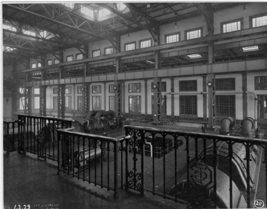
Fig. 7 Interior Sala turbinas 1927
