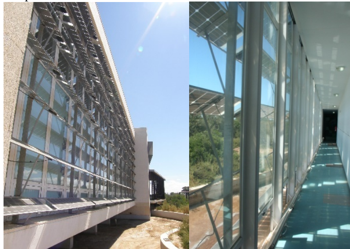
Fig. 9 Solar panel. View from the inside and the outside of the building.
