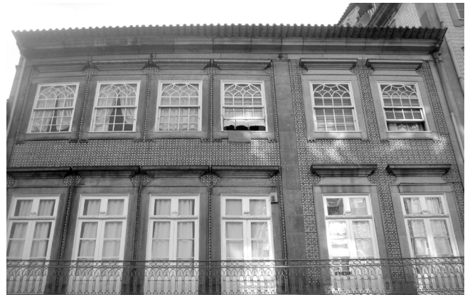
Figure 2. Main street façade of Model M1: First floor – Casement Windows: Cw.1 and Cw.2; Second floor: Sash Windows Sw.3, Sw.4
