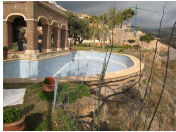
Fig 8 "Landslide" and Fig 9 "Landslide"
