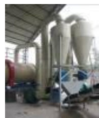
Cyclone collects dust while removing dried material
