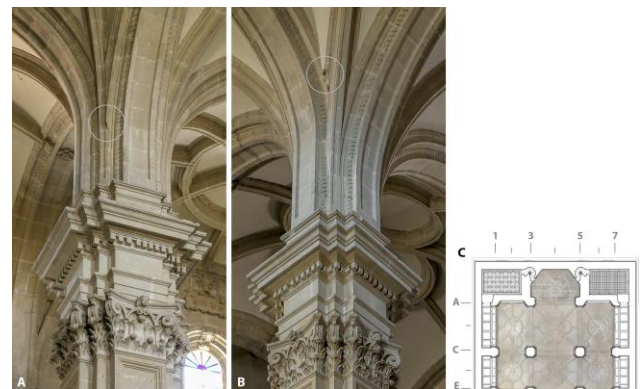
Fig. 12: (a) Detail of an abrupt interruption in the rib mouldings, (b) detail of a scroll on a diagonal rib and (c) site plan
