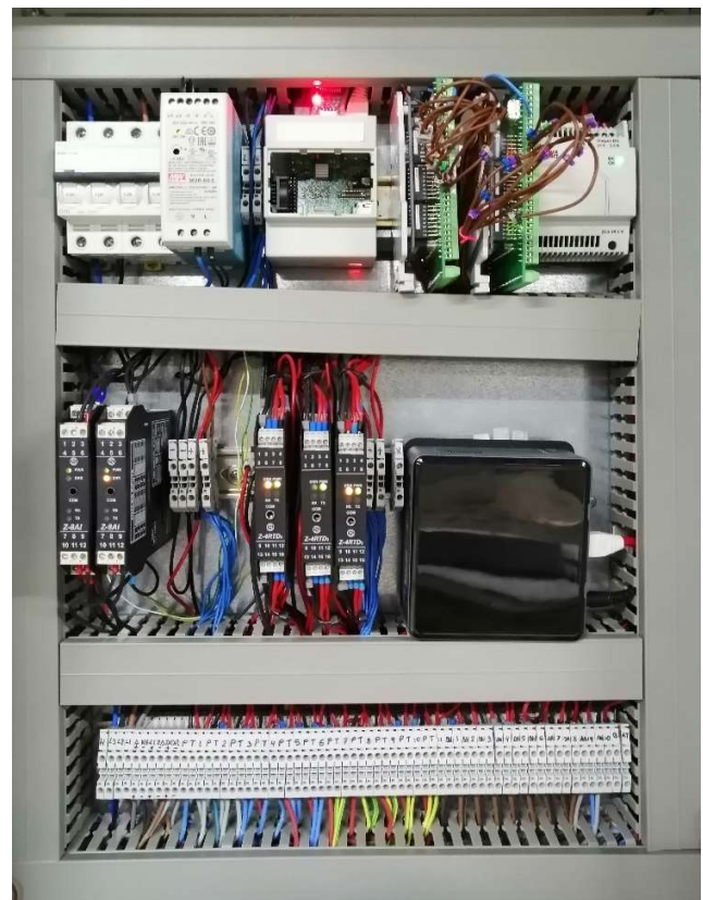
Fig. 9. Real installation in an electric box inside the chilled water pumping room
