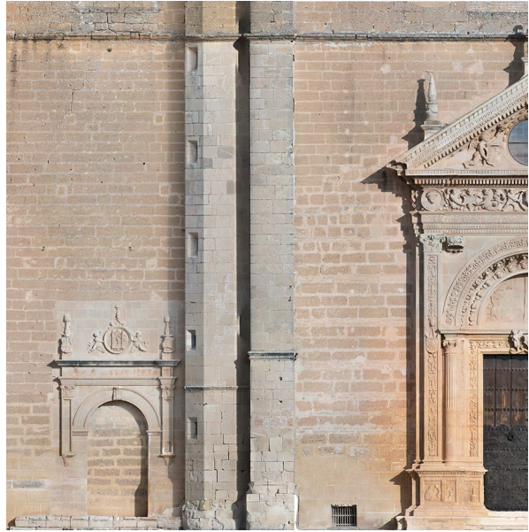
Fig. 11 Orthophoto (fragment) of the facade of the collegiate church of Osuna. Image: Fernando Díaz Moreno and Eduardo Acosta
