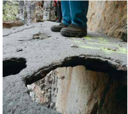
Figure 3. Previous state of the footbridge. Source: Machuca Santa-Cruz, Luis (2016). "Recuperación del Caminito del Rey".
