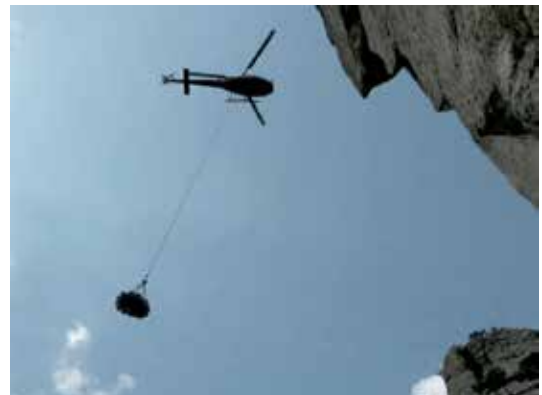
Figure 12. Helicopter delivery of materials and waste management for greater precision and efficiency.
