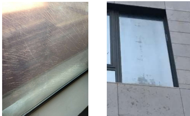
Figure 4. Examples of windows of the building considered in this study with the damaged SCF
