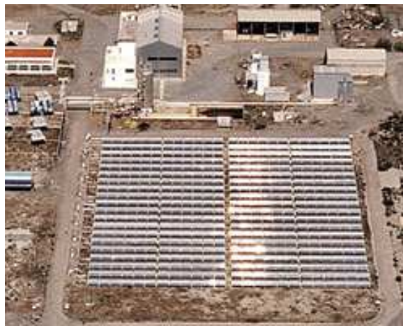
Figure 2.2: DISS solar plant.
