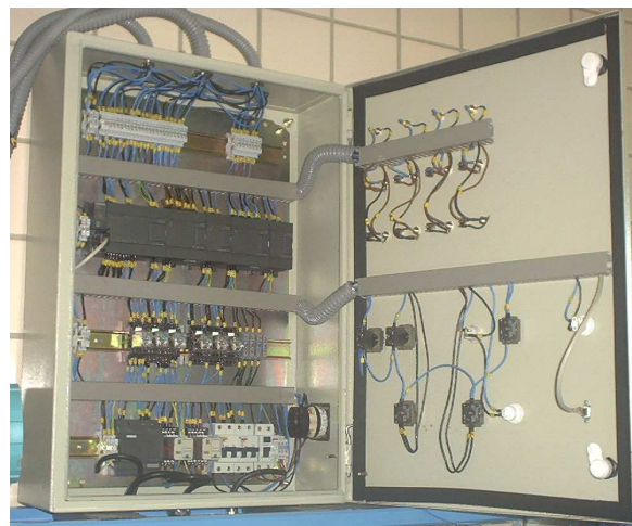
Figure B.5: Electric panel
