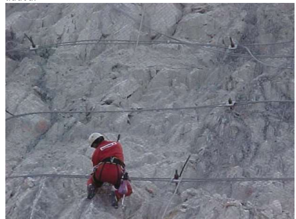
Figure 4. Tecco mesh reinforced by cables (courtesy of Geobruigg)
