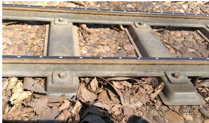
Figure 9. Track railhead marking
