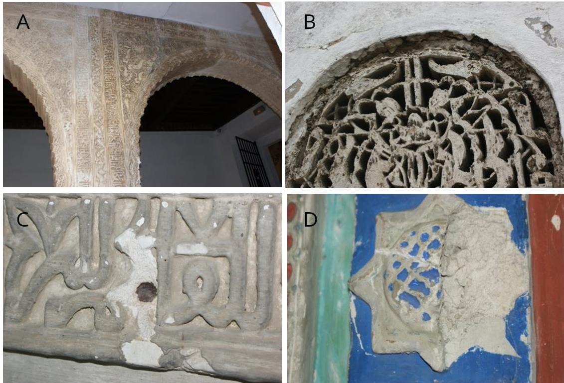
Fig. 4 Deterioration in RAS plasterwork: water seepage (A), direct action of rain (B), detachment after oxidation of the metallic element (C), disintegration of the material (D).
