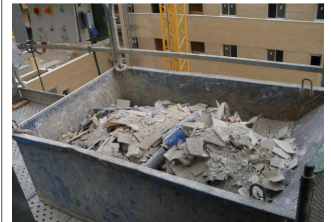
Figure 1. Waste of building elements separated and piled on the place of work or in containers.
