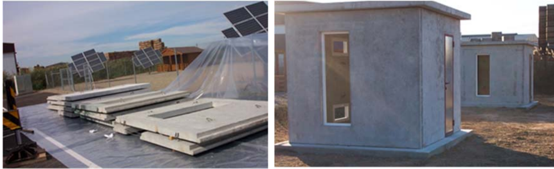
Figure 1. Construction of the cubicles with prefabricated concrete panels in 2005 at the experimental setup of Puigverd de Lleida (Spain)
