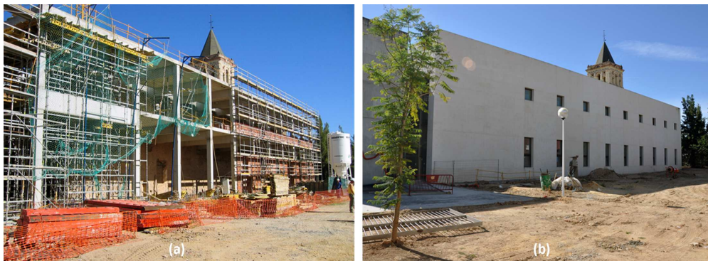
Figure 2: Views of the civic center (a) under construction (2012) and (b) in service (2013).
