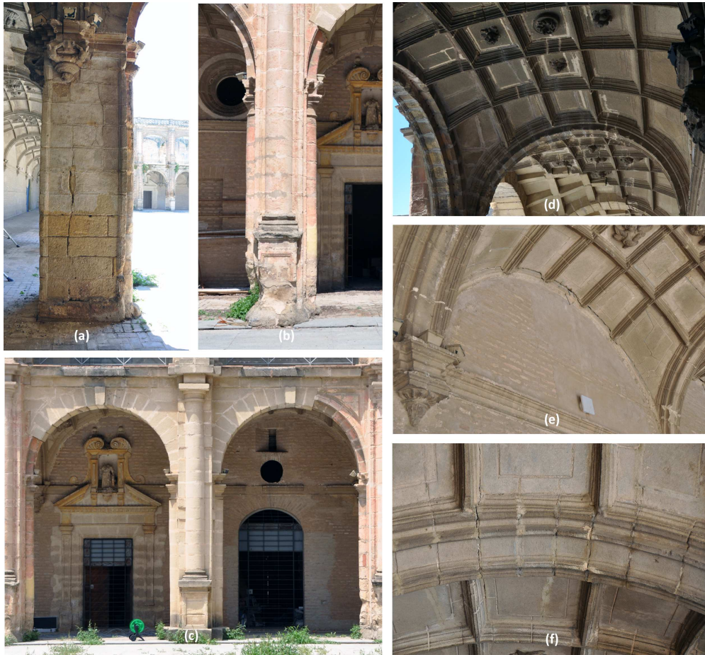
Figure 6: Most significant damage: (a) vertical cracks in the north wing columns; (b) section loss in the north wing columns; (c) rebuilt column after the 1969 Portuguese earthquake (Fig. 9 - column 10); (d) longitudinal cracks in the vaults of the ground floor of the north gallery; (e) Longitudinal cracks at the intersection of the vaults with the historic wall of the east wing; and (f) cracks in the keys of the arches of the ground floor of the east wing.
