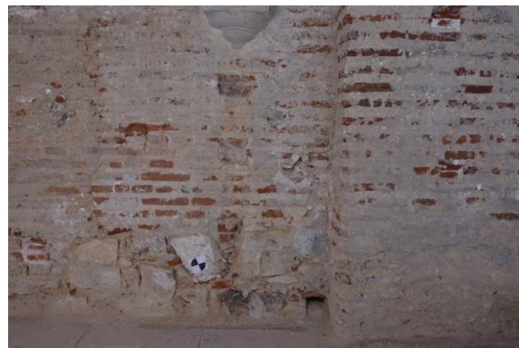
Figure 13. Detail of the facing of the church, the original wall and the reforms of the Cloister
