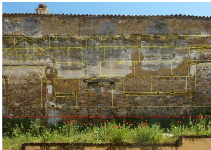
Figure 16. North facing 2, with the elements of the south face, georeferenced and indicating the original floor level of the cloister
