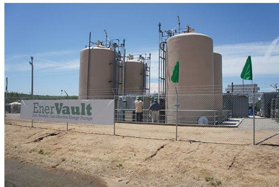
Figure 2.4 1 MWh- equivalent tanks [48].
