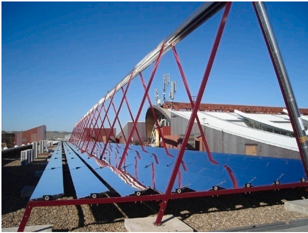
Fig. 2. Fresnel-type solar field.
