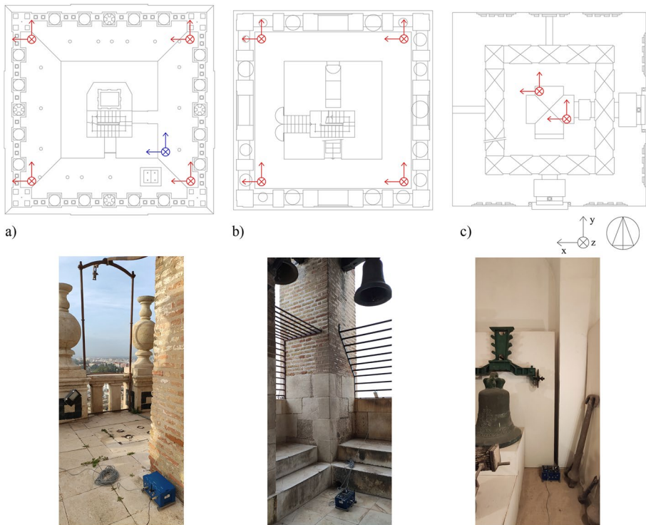
Fig. 6 Location of the triaxial accelerometers for the ambient vibration test: a rooftop, b belfry and c 6th floor room. The sensor fixed has been depicted in blue and the different measurement set-ups in red
