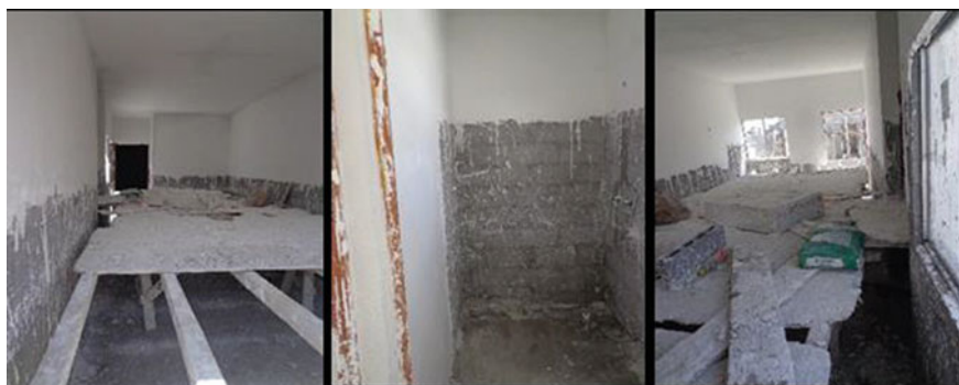
Fig. 5 Inner plaster finish and reinforced concrete vault block concrete slab. Source The authors
