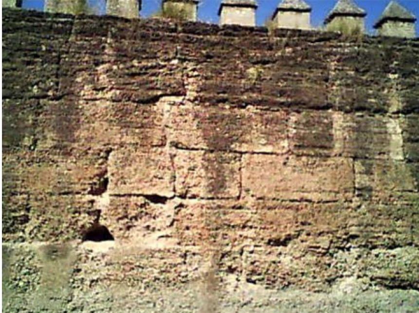
Figure 1. Biological degradation in the Macarena wall.
