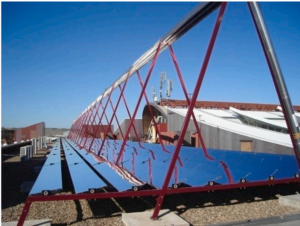
Fig. 1. Fresnel solar collector installed at ETSI absorption solar plant [34].
