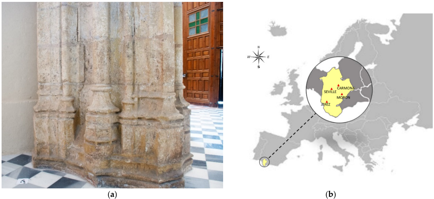
Figure 1. (a) Photograph of the pillar of the church in Morón de la Frontera. (b) Location of Seville cathedral and other gothic churches.
