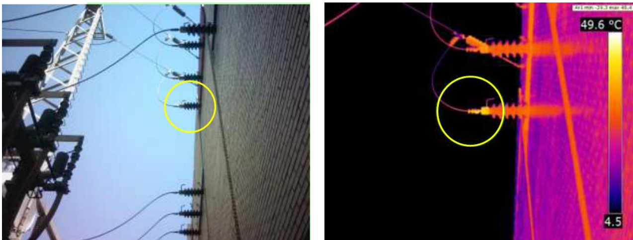
Figure 2. Visible and infrared images of a hot spot in a 66 kV wall bushing connector.
