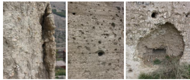
Figures 23, 24 and 25. Loss of whitewash as a result of internal wall washing, shrapnel marks and the presence of plant organisms are shown in sequence. Photography: Félix Pérez Moreno and Jorge Moya Muñoz 2019.
