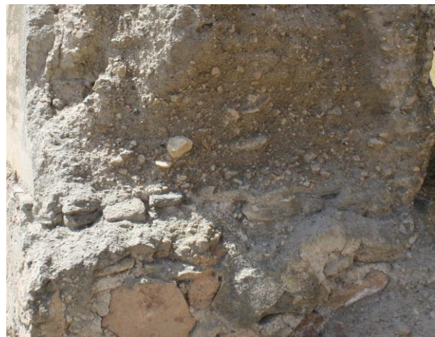
Figure 14. Wall section view: the layer of stones for the regularisation of the rammed-earth wall on the top can be observed. The whitewashing, the interior material components and the aggregates measure used can also be seen. Photography: Jorge Moya Muñoz 2019.
