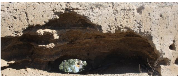
Figure 6. Loss of mass and wall section in north side of the 'Alcazaba' rammed-earth wall. Photography: Jorge Moya Muñoz 2019.
