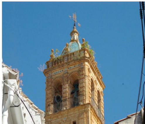
Figure 9. Detail of the current state of the dome.
