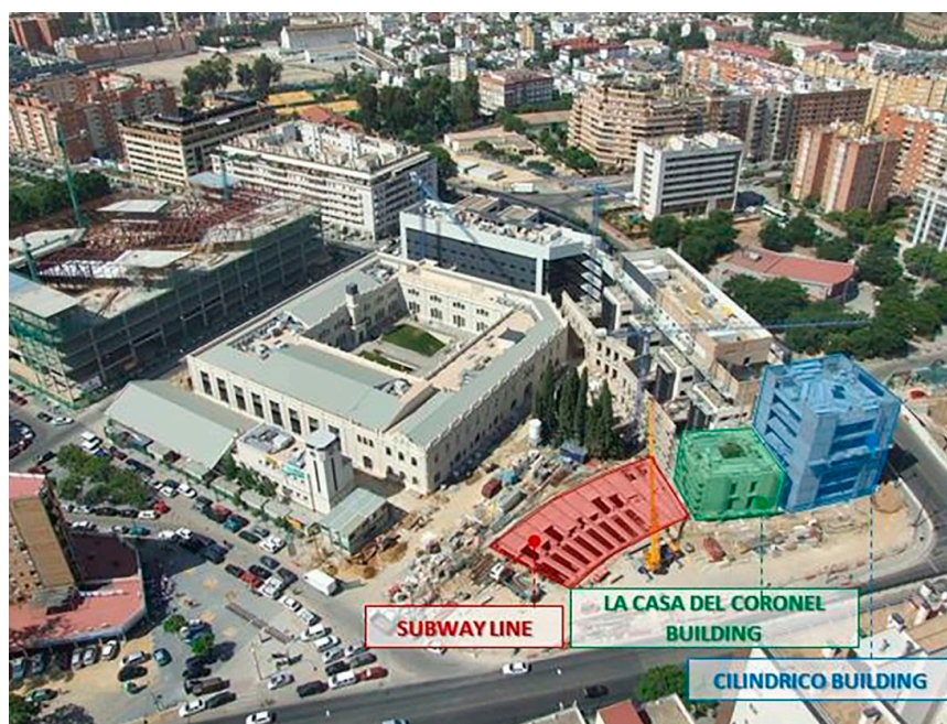
Figure 2. Execution of the works on the Cilíndrico and Casa del Coronel buildings over the Seville subway line. Source: The authors.
