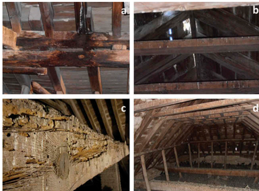
Figure 7. (a) A fungus infection of the timber roof could be due to permanent damp, dirt collection and natural causes; (b) external atmospheric actions (strong wind and rainwater); (c) active attack of xylophages' insects; and (d) Biological actions inside the roof.
