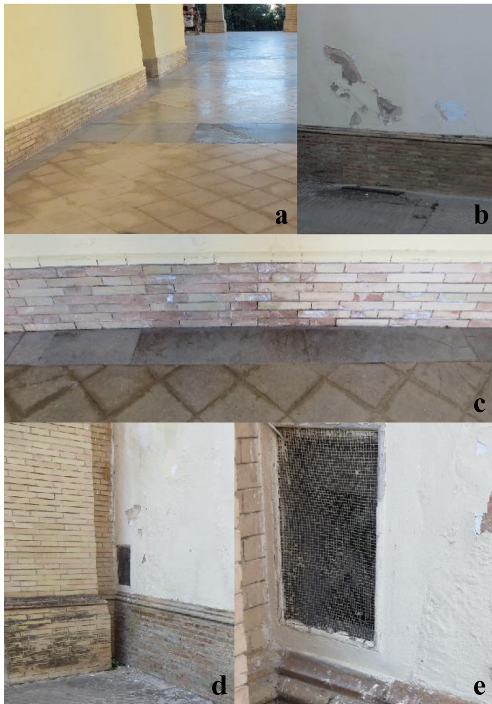
Fig. 8. Pathology observed in the building mainly due to raising damp.
