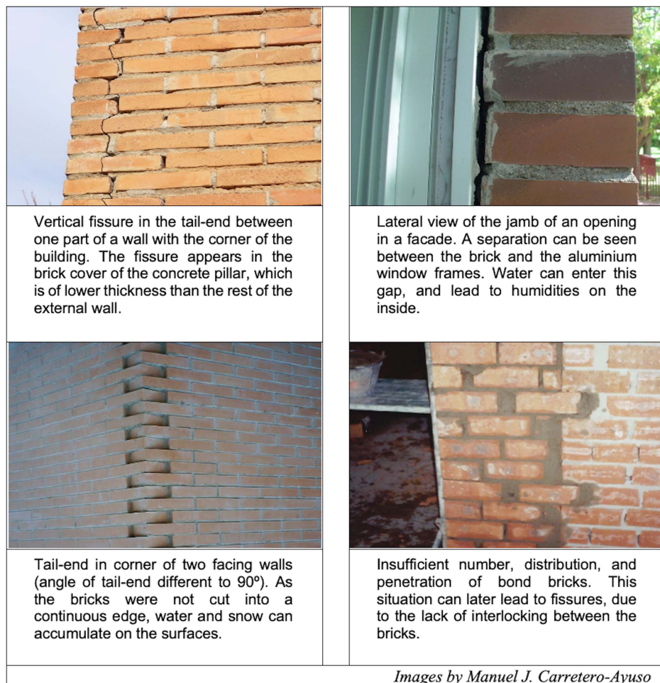
Fig. 5. Photographic examples of several execution problems.
